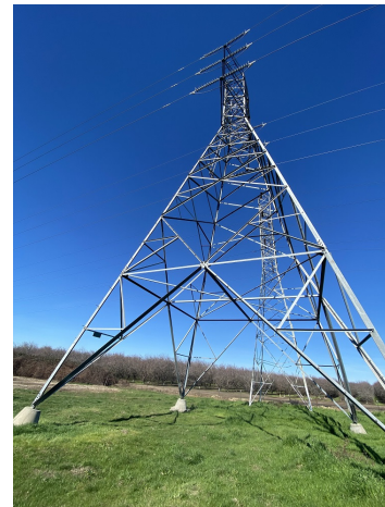
Transmission Line 7/8 Tower 508S Looking North
