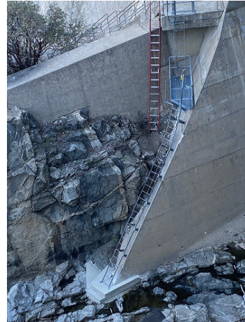
Spillway Access Ladder with Fall Protection
