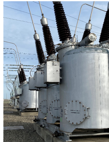
Oil Circuit Breakers
