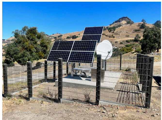
ACDD VSAT Enclosure complete with new solar system
