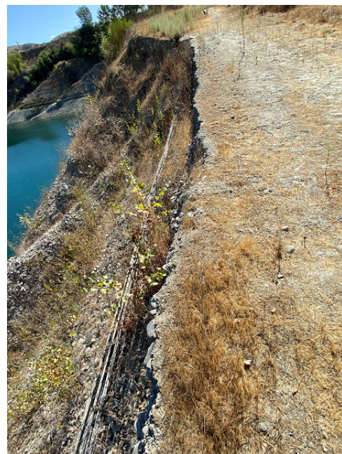
Erosion Along Access Road
