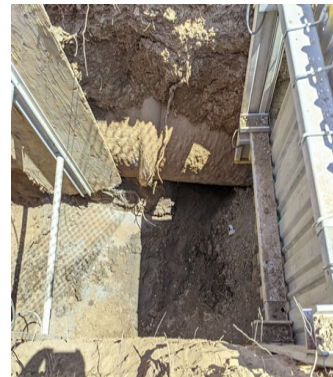
Void beneath pipeline discovered during leak investigation
