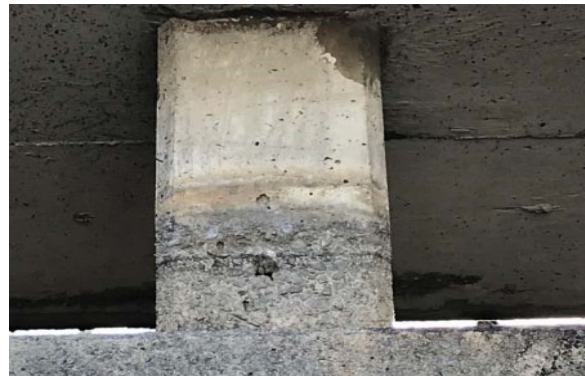
Concrete Scaling within SVWTP Sedimentation Basin to be Repaired by Project
