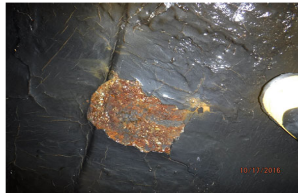
Typical coal tar lining failure
