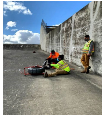
Spillway drain inspection crew inserting camera for visual inspection of drain holes
