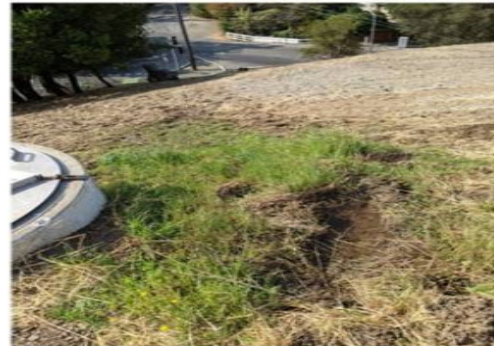
Location of leak on BDPL4 PCCP in Redwood City
