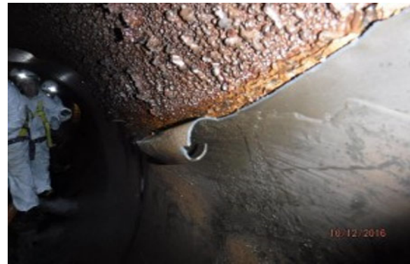
Lining Disbondment and Scaling
