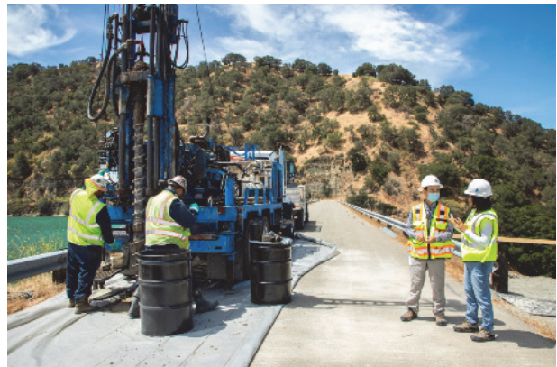
Crews performing geotechnical drilling work on dam crest during DSOD site visit
