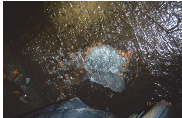
Typical lining failure
