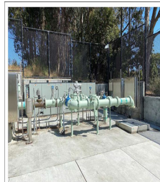
Typical well station equipment
