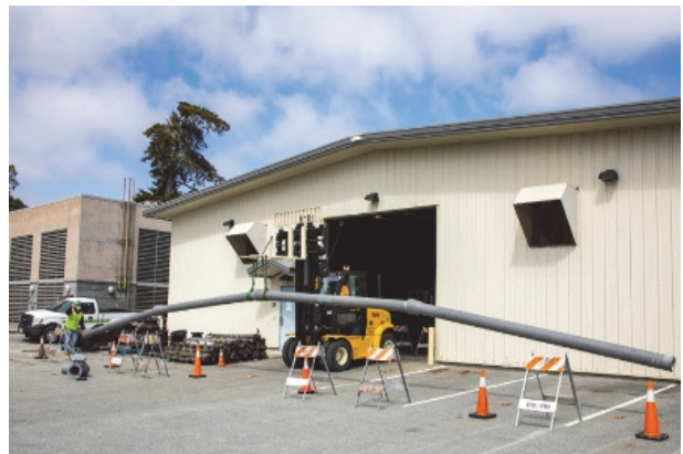
Earthquake Resistant Ductile Iron Pipe with flexible joints (demonstrated) used for this project
