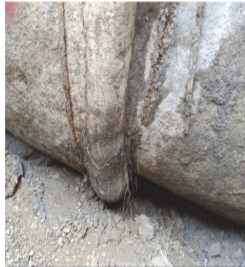
Leak at PCCP to Steel Transition
