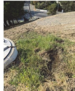
Location of leak on BDPL4 PCCP in Redwood City
