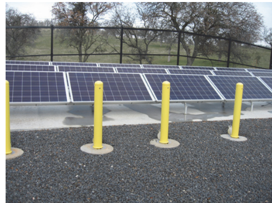
Oakdale Valve House No. 4 Solar Facilities
