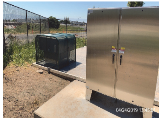
Ventilation Fan and Control Panel at the Articulated Vault
