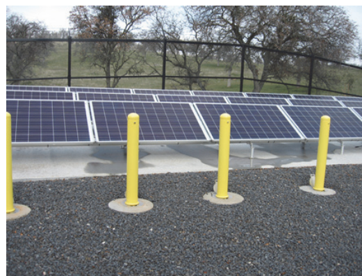
Oakdale Valve House No. 4 Solar Facilities
