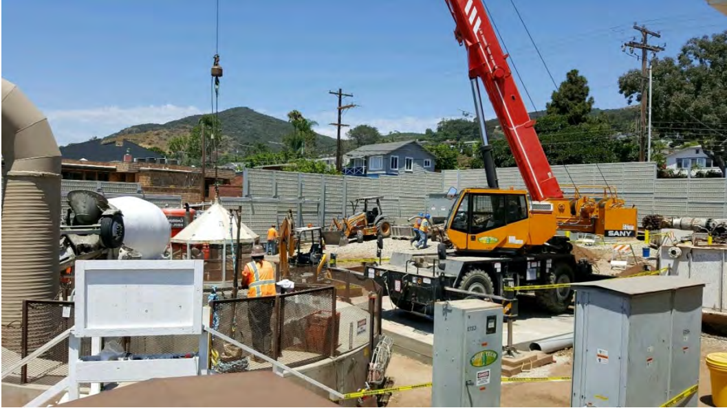
Figure I-4 Examples of Temporary Sound Barriers
