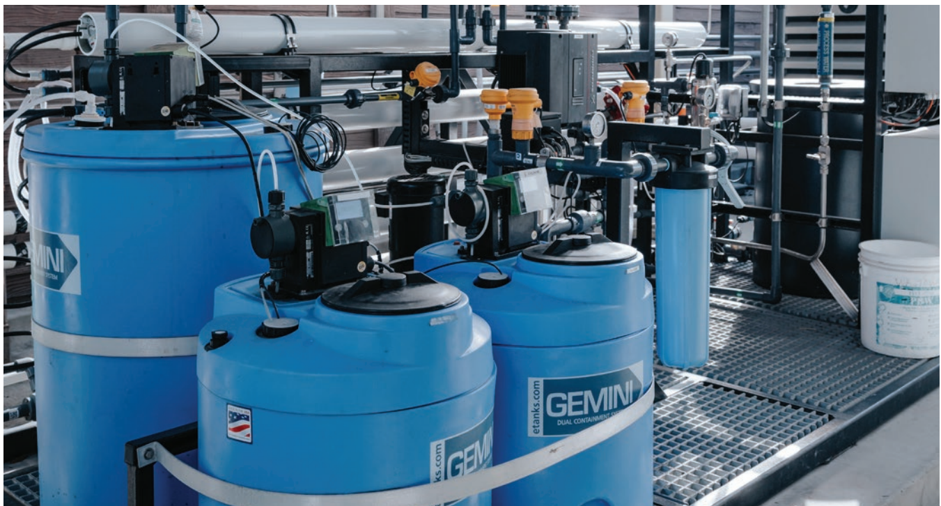
Treatment system RO skid (image courtesy of Seismic Brewing)
