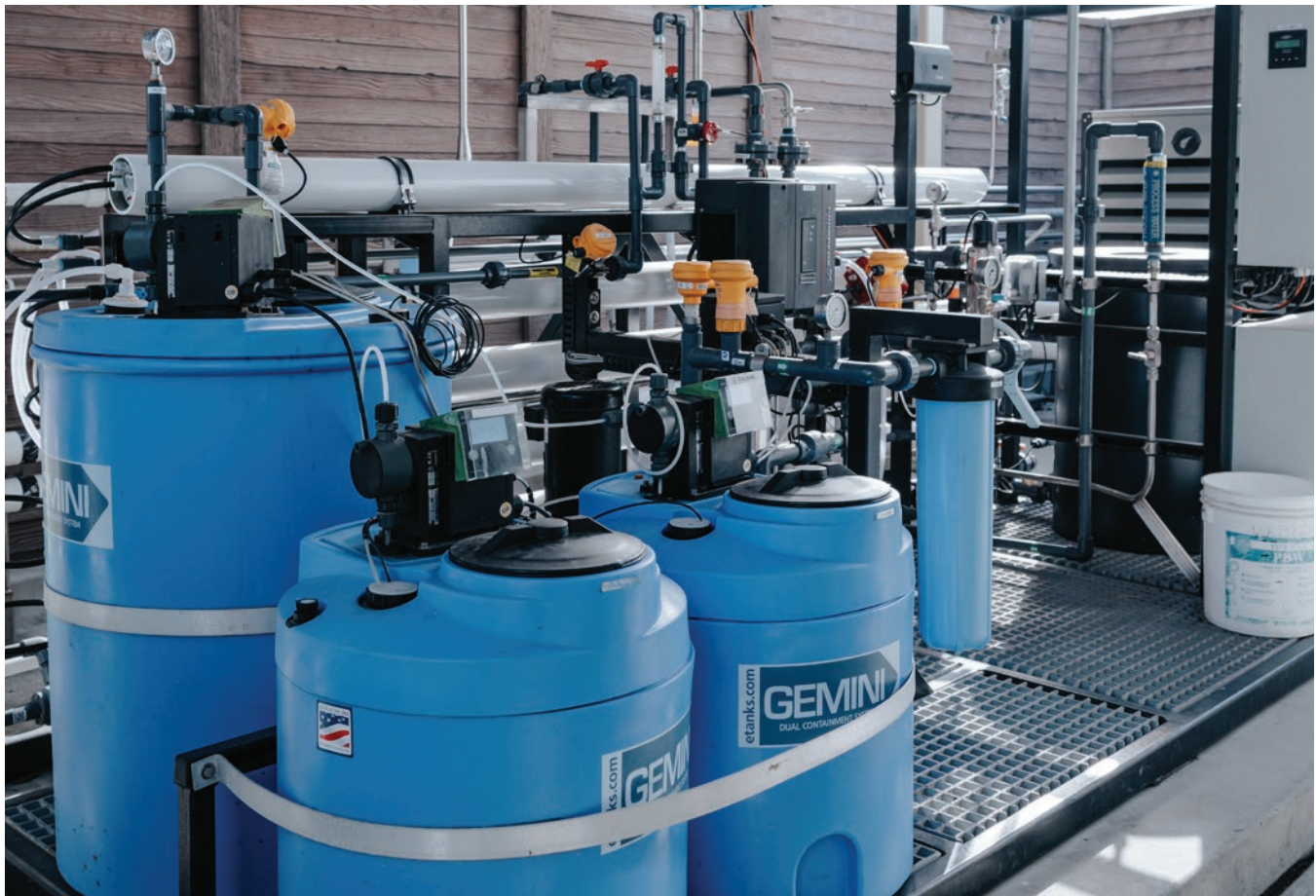
Treatment system RO skid (image courtesy of Seismic Brewing)
