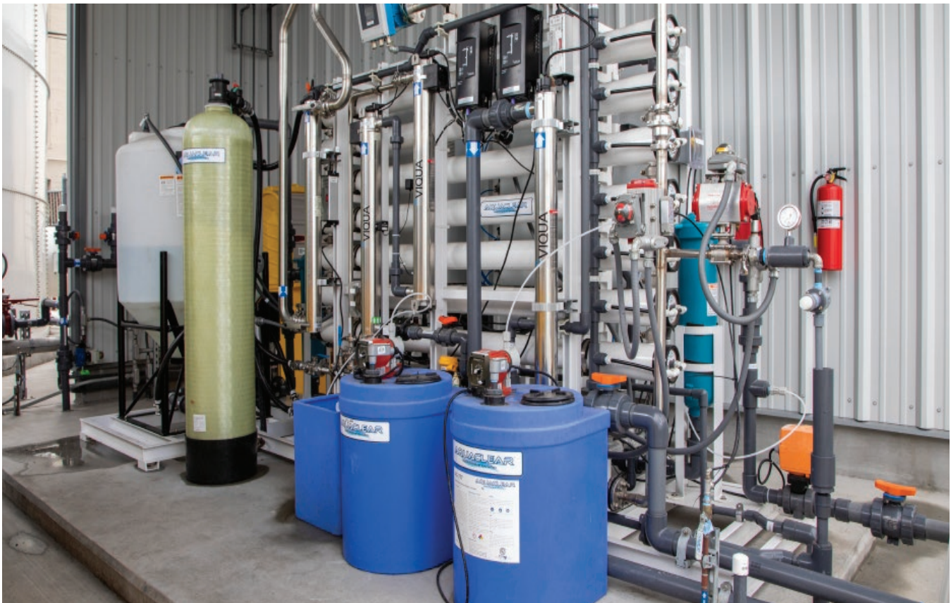
Anchor Brewing Company's brewery process water recycling system
