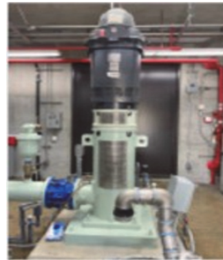
Typical Well Pump
