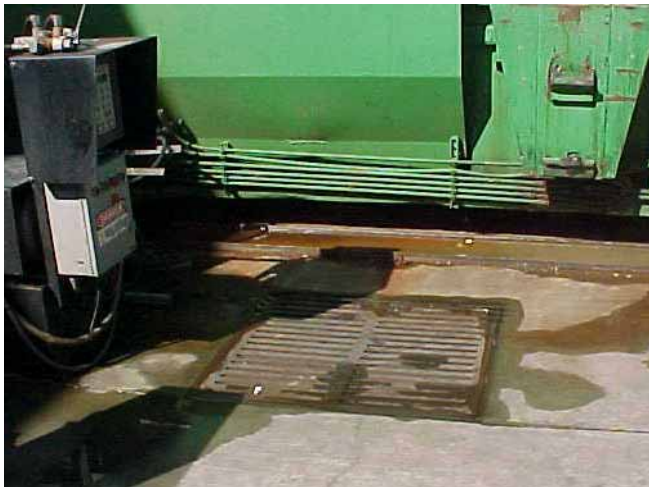
A drain adjacent to a trash compactor is connected to the sanitary sewer system. A concrete berm surrounding the trash storage area hydraulically isolates stormwater runoff in this area from the rest of the site.
