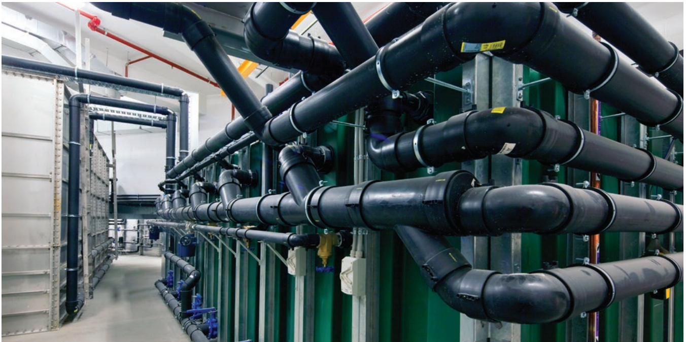
An onsite reuse system (image courtesy of Aquacell)
