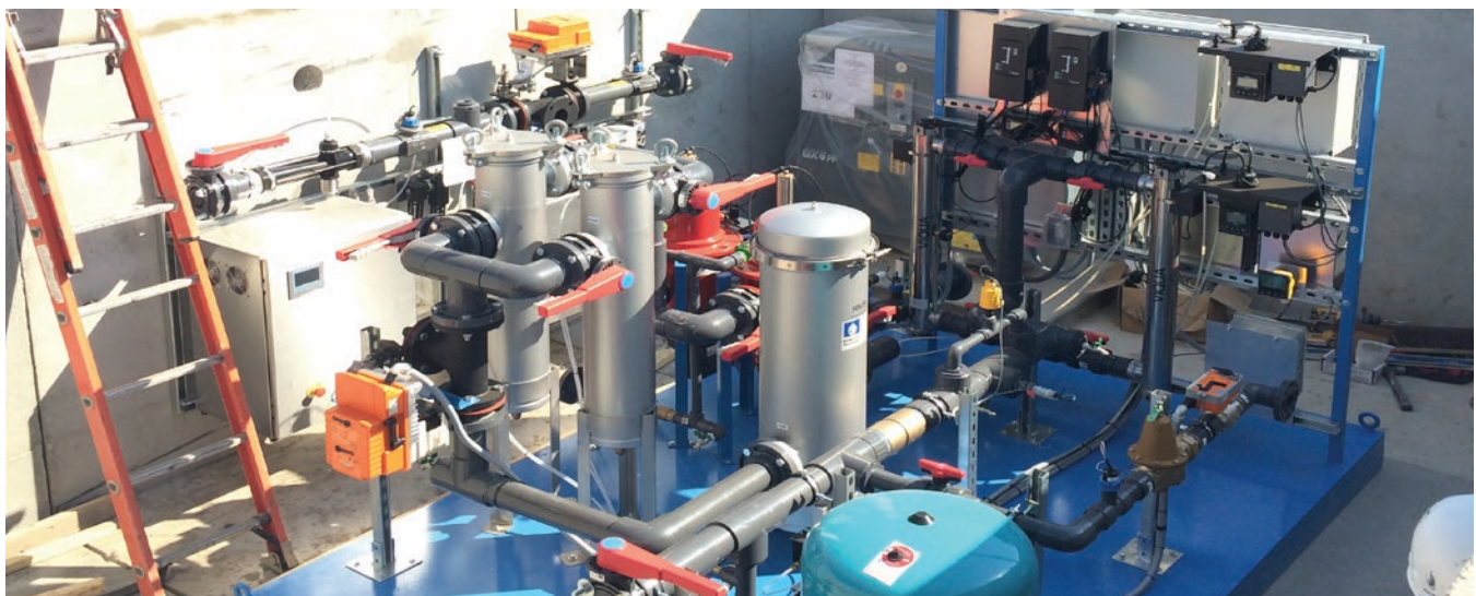
Onsite reuse system's "Smart Hub" (image courtesy of the City of St. Paul)
