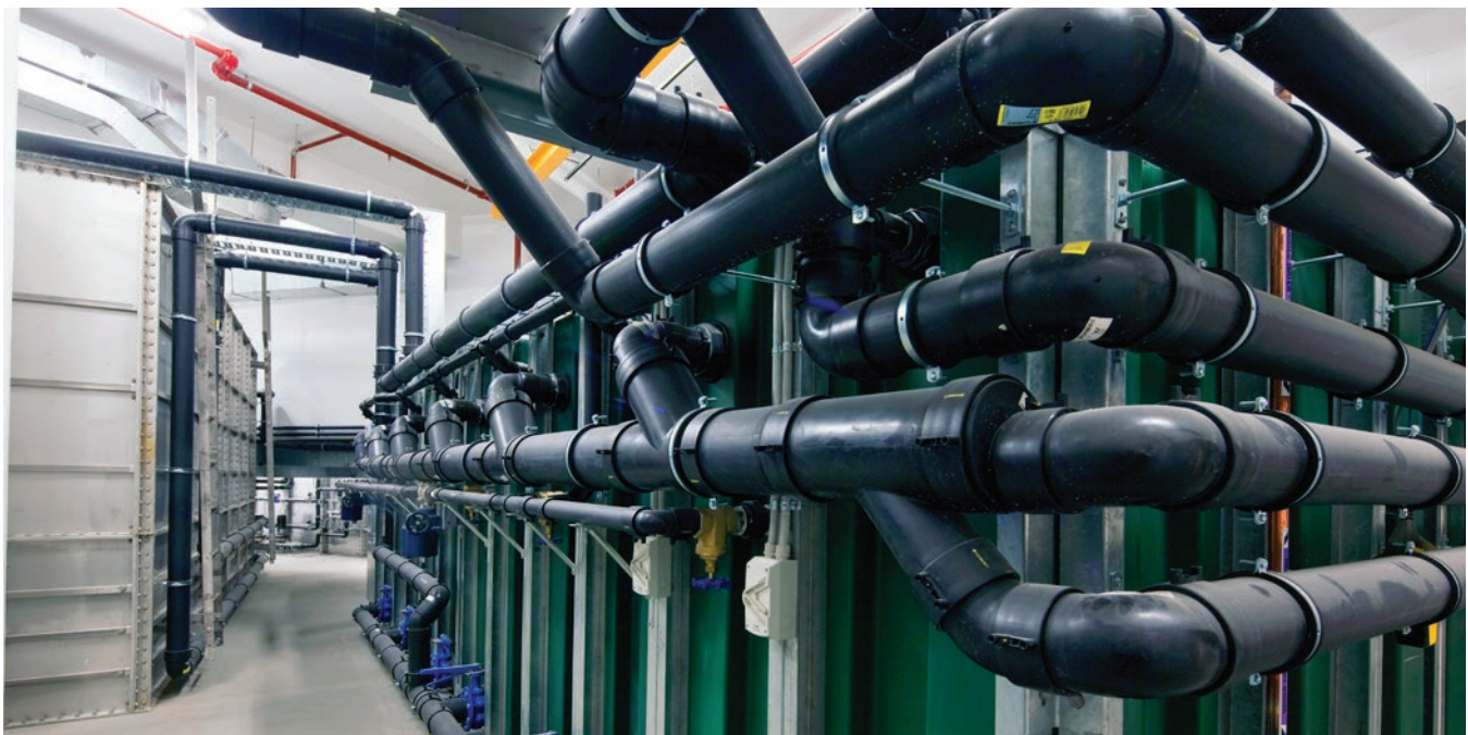
1 Bligh Street's onsite reuse system (image courtesy of Aquacell)
