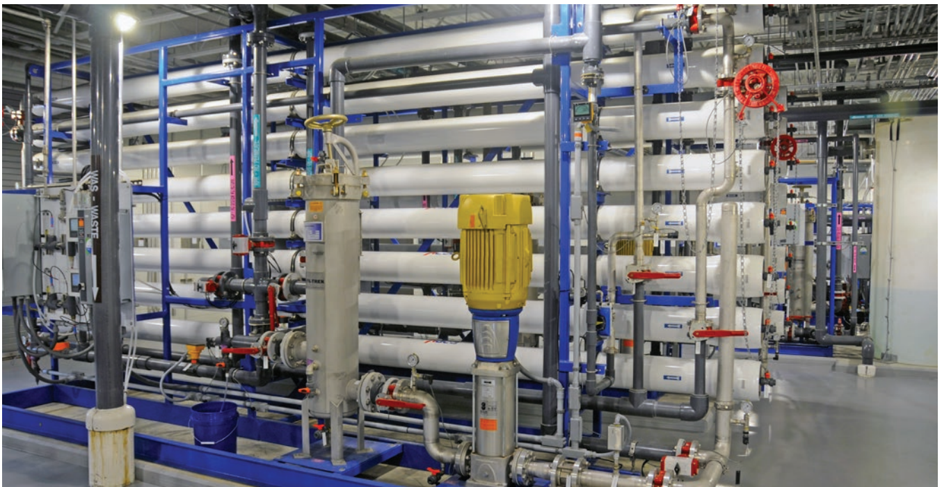
An onsite reuse system's mechanical room (image courtesy of Sustainable Water)
