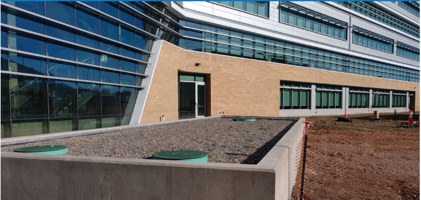
3rd stage of wetland treatment during its construction on the roof (image courtesy of Denver Water)
