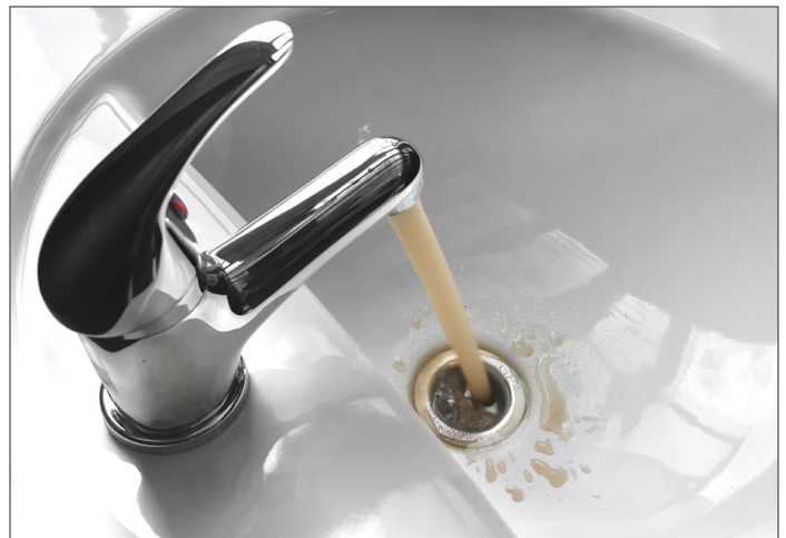
Discolored water from faucet after a water main break.
