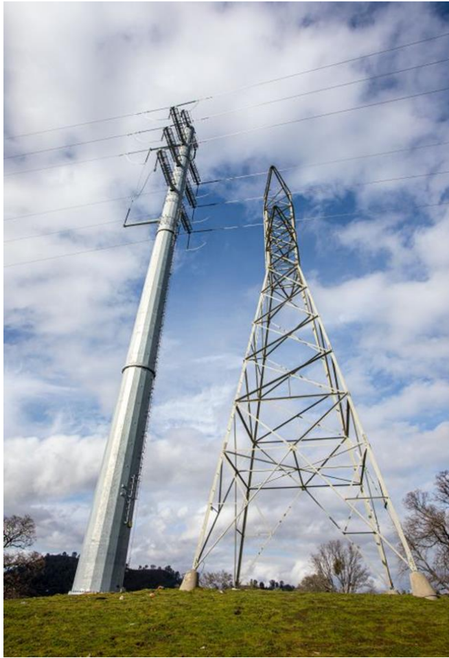
Transmission tower, power lines at Don Pedro Reservoir
