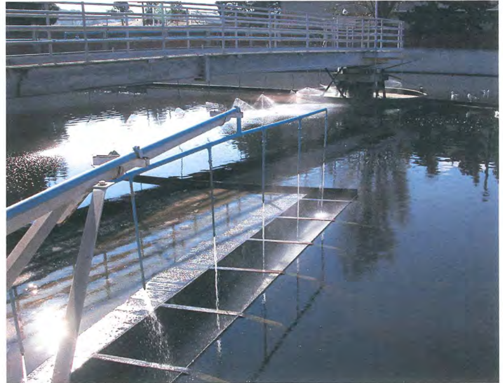
Clarifier at Southeast Treatment Plant
