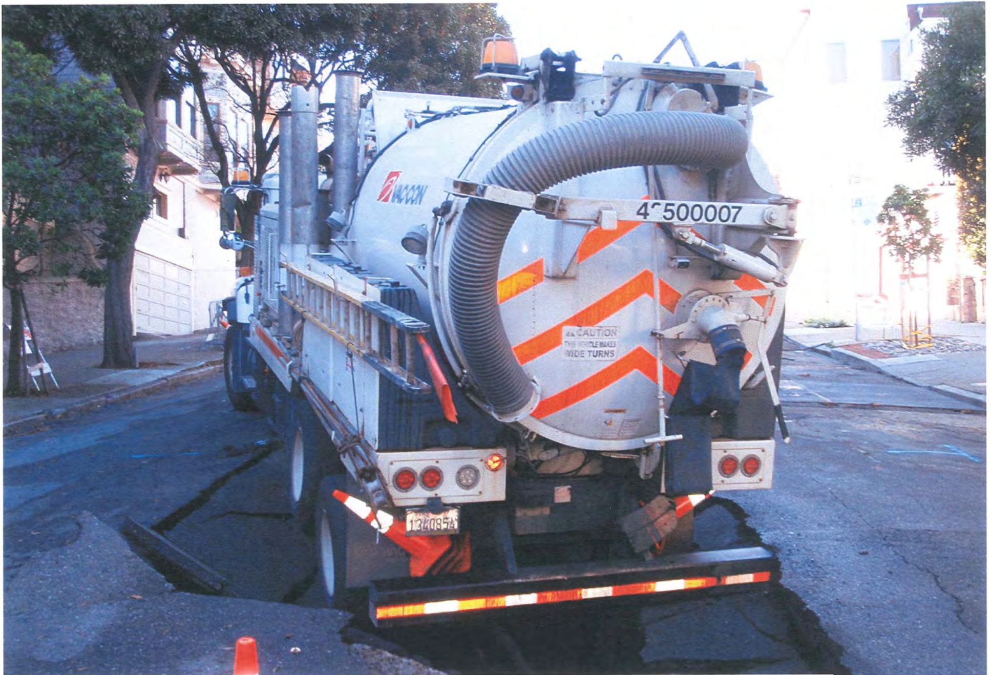
Our Sewer System is Aging and Failing: Waller St. at Divisadero St.
