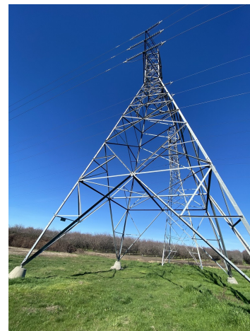
Transmission Line 7/8 Tower 508S Looking North
