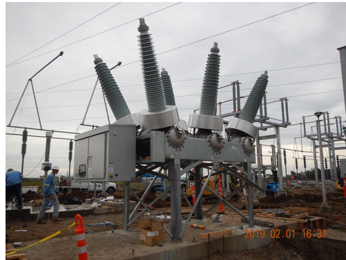
Typical 230KV SF6 Breaker to be Installed as Part of Phase II
