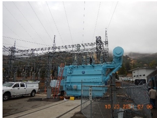
Delta Star GSU1 Transformer in Spare Slot
