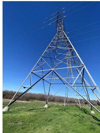
Transmission Line 7/8 Tower 508S Looking North
