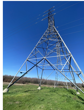
Transmission Line 7/8 Tower 508S Looking North
