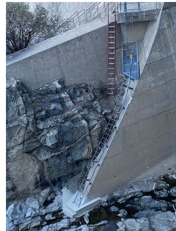
Spillway Access Ladder with Fall Protection
