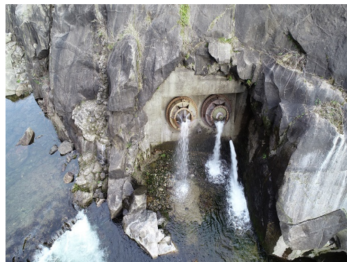
O'Shaughnessy Dam Instream Flow Release Valves
