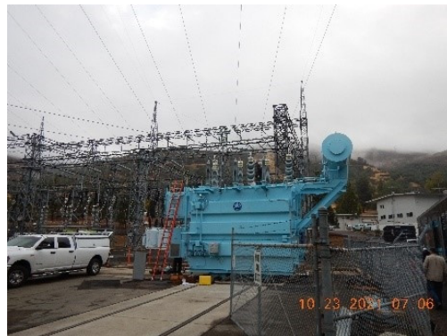
Delta Star GSU1 Transformer in Spare Slot
