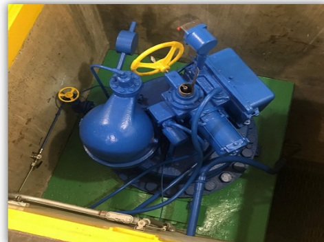
Turbine bypass valve
