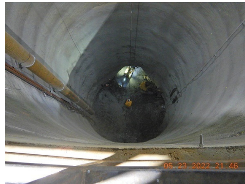
Flow Control Facility Shaft and Bypass Tunnels (View from top of shaft looking down)
