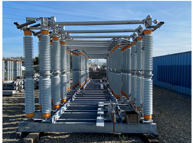
High Voltage Disconnect Switches (WSR Phase 2)
